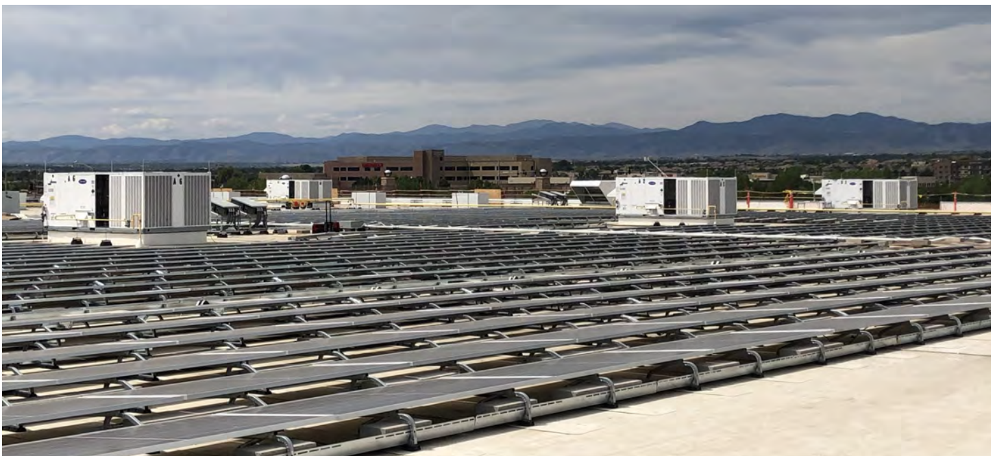
SOLAR INSTALLATION AT THORNTON CROSSING, THORNTON, COLORADO COMPRISES OVER 17,000 PANELS COVERING 19 ACRES OF ROOFTOP
